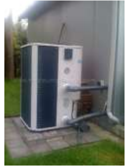
A 20 watt heat pump unit in Essex
