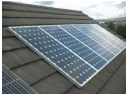
Solar panels are increasingly used to provide heat in houses
