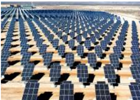
A huge solar power plant in Nevada
